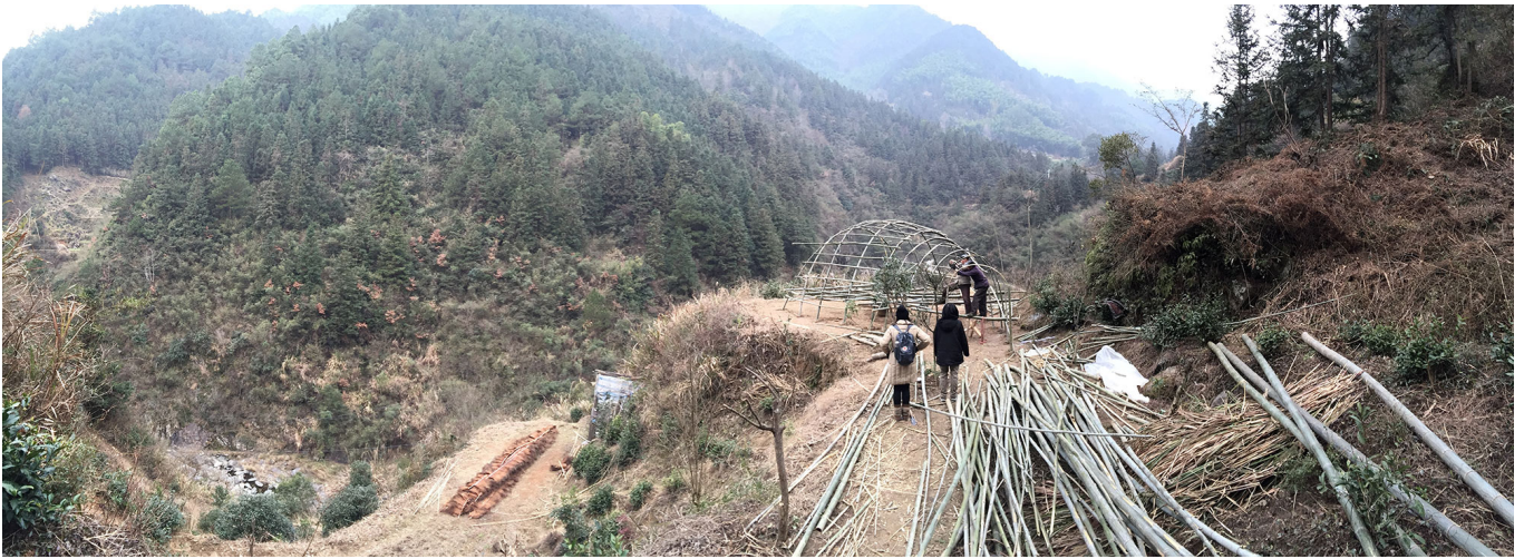
A hand-built bamboo tea house “Happiness Pavilion” in construction, January 20, 2016. The project was an architectural cooperative experiment by the villagers, Qian Shi’an, Cheng Guofu, Chu Chunhe, and Ou Ning. Photo: Ou Ning.
