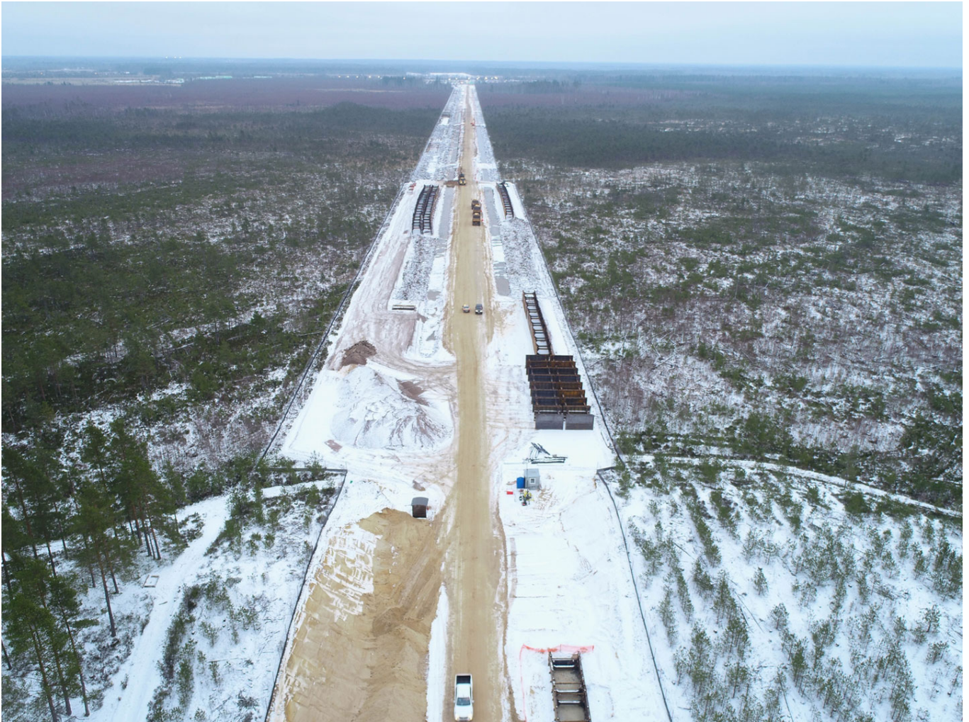
Construction corridor for the Russian onshore section of Nord Stream 2 pipeline. Copyright: Nord Stream 2 AG / Agiteco.
