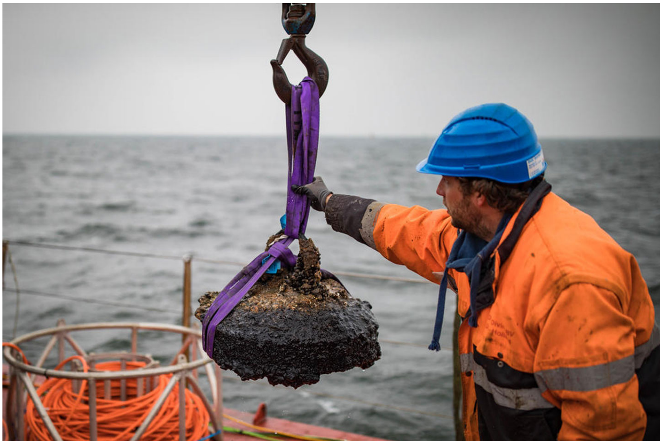
A munitions clearance operation on the Nordstream 2 pipeline route, which runs in close proximity to World War II chemical weapons dumping grounds. Copyright: Axel Schmidt.
