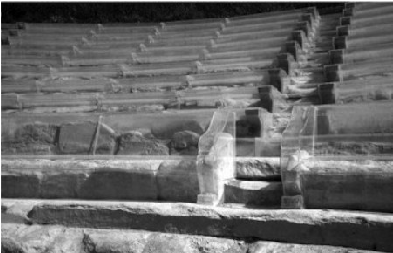
Supplemental plexiglass seating over the original stones of the Greek Theater at Heraclea Minoa, Agrigento, designed by Franco Minissi (1960–63). Left: as built in 1973. Photo courtesy of C. Bellanca. Right: The first level of bleachers with breaking laminate and greenery infestation, 2000, (N. P. Stanley-Price, J. Jokilehto, "The decision to shelter archaeological sites: Three case studies from Sicily," Conservation and Management of Archaeological Sites no. 5, 2001: 19–34).
