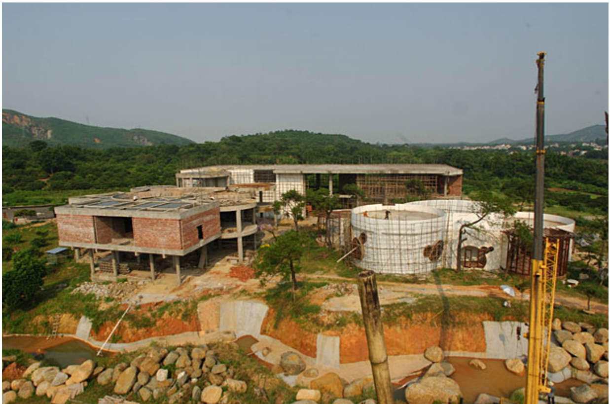
An unusual building being built at the foot of the mountain for Zheng Guogu's Age of Empire , 2009. Photo courtesy of the artist.
