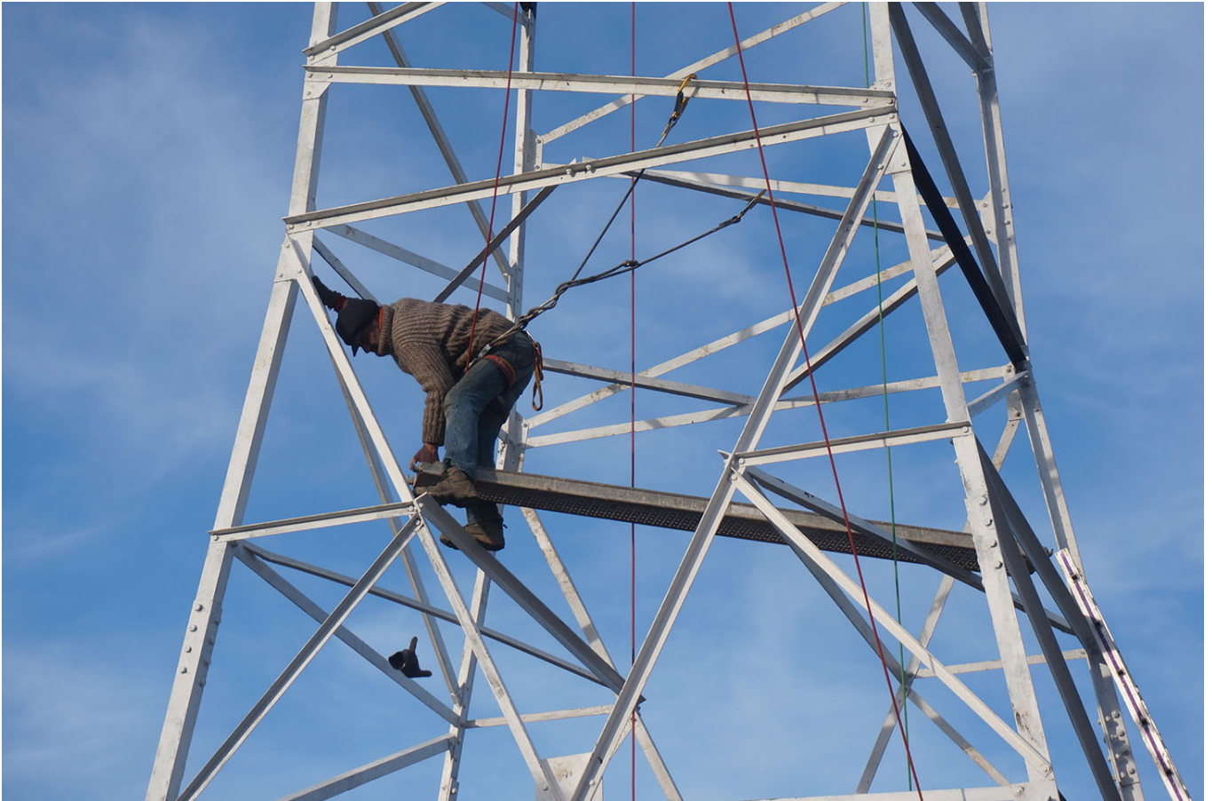
The construction of a lighthouse at the ZAD, Notre-Dame-des-Landes, France, 2017. Built by farmers, boat builders, artists, and activists, the lighthouse is on the same site where the French government wanted to put a control tower for a new airport. Photo: Jay Jordan.
